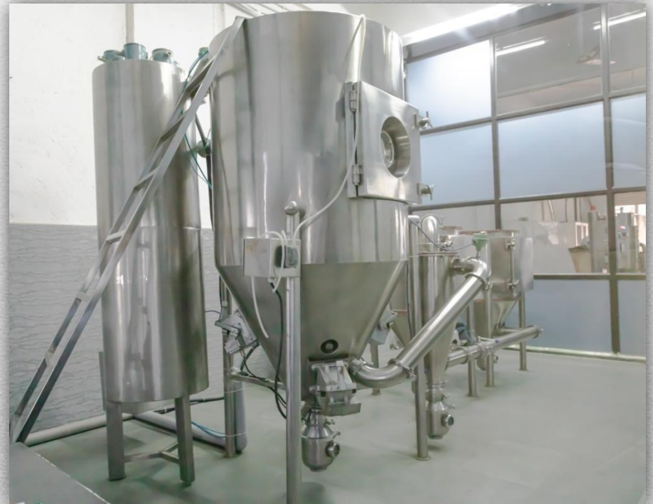
Pilot Trial Facility
